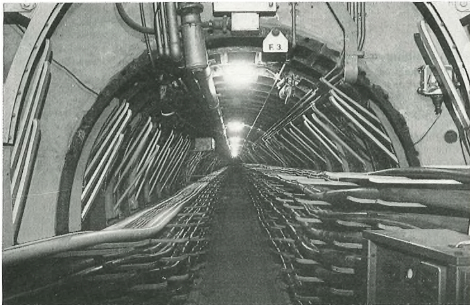
FIG. 2—Typical 7 ft diameter cable tube approximately half-filled
