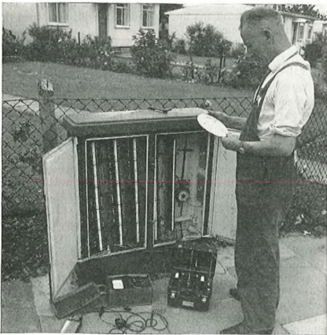
FIG. 4—Using Ohmmeter No. 18A and fault-locating slide-rule
