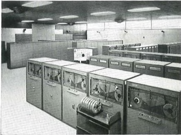
Magnetic tape units in foreground. Conditioned air is supplied by ceiling diffusers
