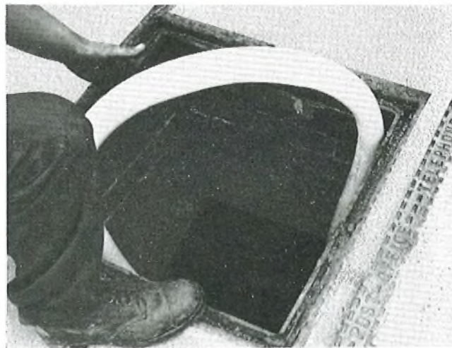
CENTRE OF THE BIGHT OF 1,800 PR., 4 LB/MILE POLYTHENE UNIT-TWIN CABLE ENTERING THE MANHOLE
