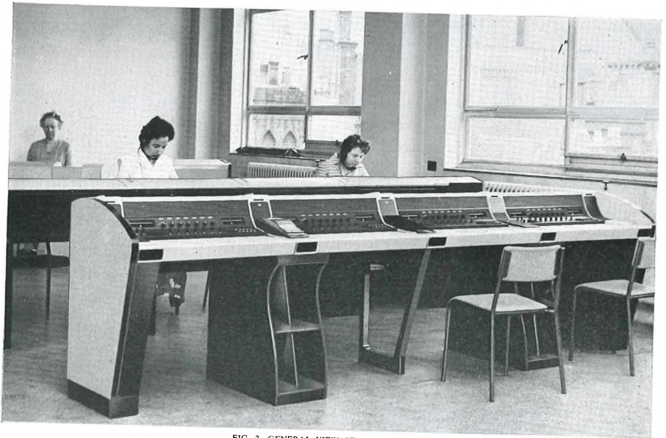
FIG. 2—GENERAL VIEW OF SWITCHROOM
