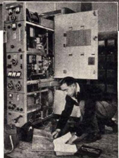
A member of the New Zealand P. T. & T. staff making adjustments during installation.
