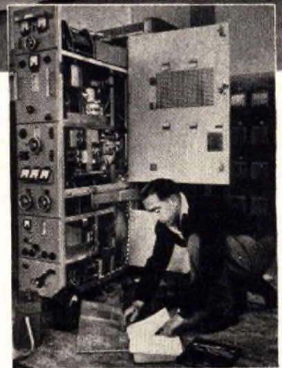
A member of the New Zealand P. T. & T. staff making adjustments during installation.
