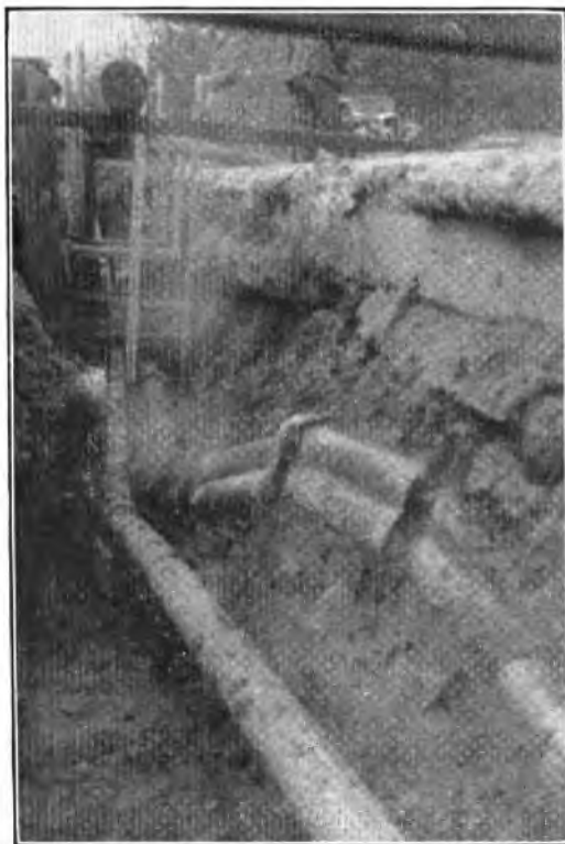
U.G. CONDUIT DISPLACED BY LANDSLIP.
