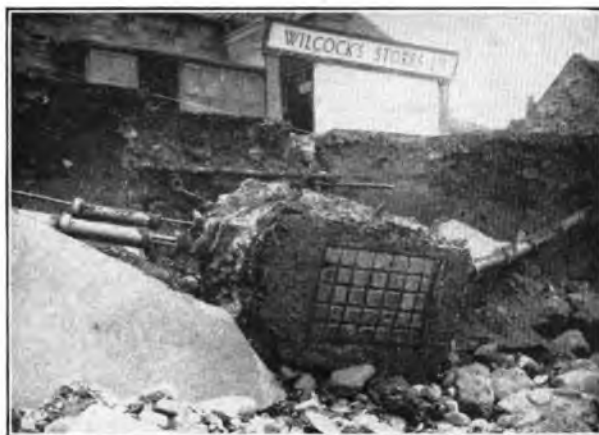
THE JOINT BOX SUSPENDED ON CABLES.
