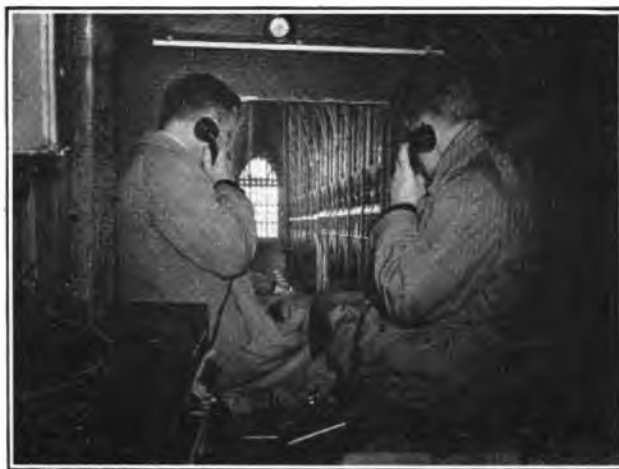
FIG. 3.—MULTIPHONE SWITCHBOARD IN CUBICLE IN TRIFORIUM.
