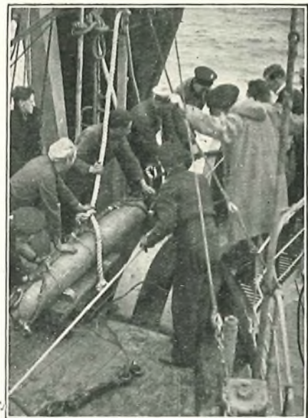
THE REPEATER AT THE STERN SHEAVE.
