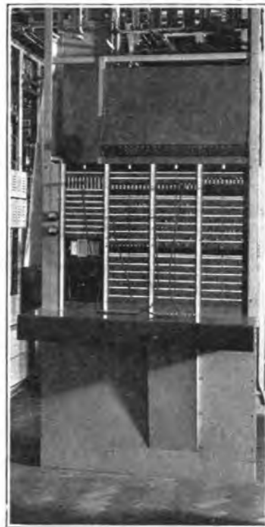
FIG. 2.—THE ENGINEERING CONTROL BOARD.
