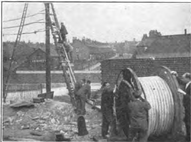
RAMP CONSTRUCTED ON SHEFFIELD SIDE; DRAWING THROUGH OF 3RD CABLE IN PROGRESS.
