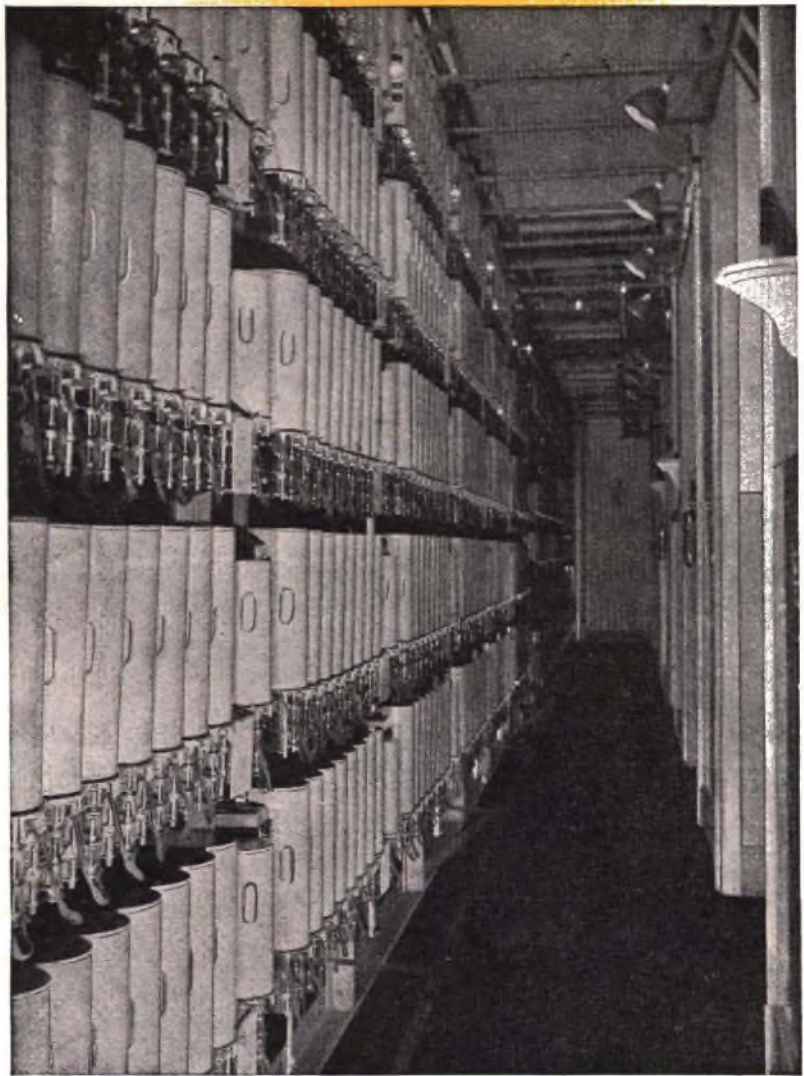
Photo: Final Selector Rack, Lisbon Exchange
