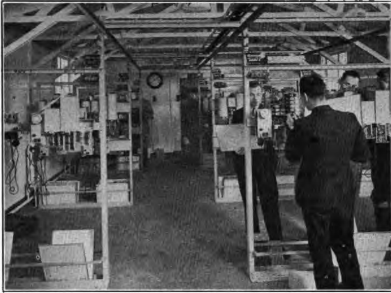
FIG. 5.—FAULTING ROOM FOR AUTOMATIC EQUIPMENT.
