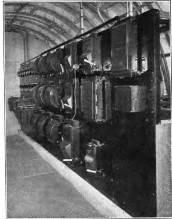
FIG. 3.—MAIN LIGHTING AND POWER DISTRIBUTION BOARD IN TELECOMMUNICATIONS TUNNEL.
