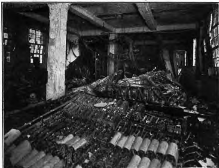
FIG. 2.—SELECTOR RACKS. THIRD FLOOR.
