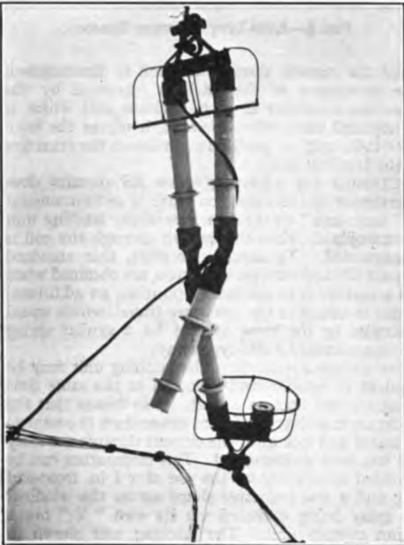
FIG. 3.—BROKEN MAIN INSULATOR ASSEMBLY.
