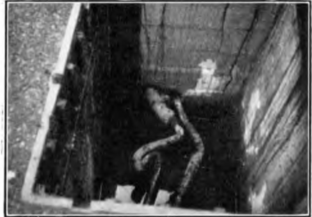
FIG. 2.—VIEW OF MANHOLE WHERE CREEPAGE HAS OCCURRED.
