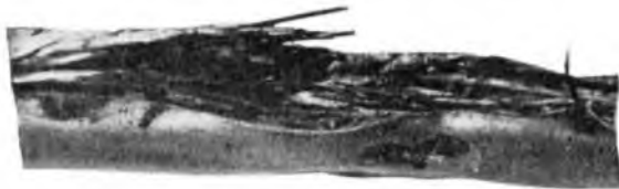
FIG. 7.—CABLE FAULT CAUSED BY LIGHTNING.
