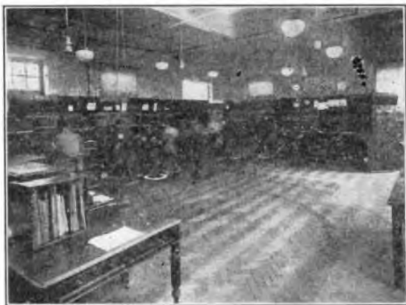
FIG. 3.—VIEW OF THE NEW SWITCHROOM.
