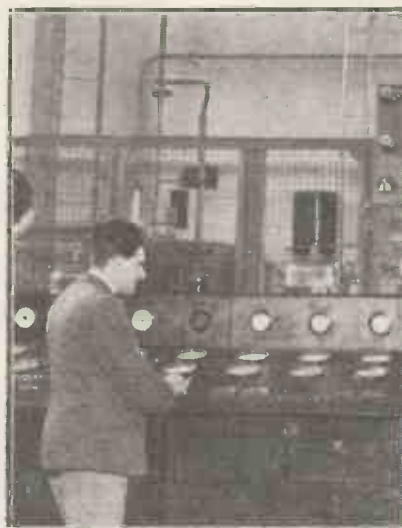
This view shows part of the control table at Rugby, the world's most powerful station, which handles all Europe's telephony to the U.S.A.
