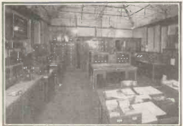
This is the control room at Savoy Hill, where the programmes must pass out from studio to transmitter.
