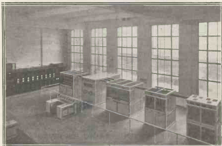
Part of the transmitter hall, showing the Regional transmitter, also the control desk and a section of the main switchboard.
