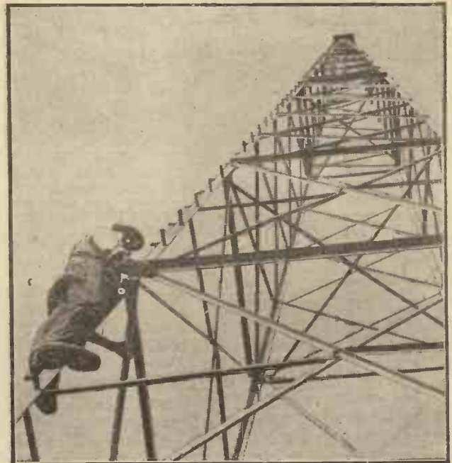
Everyone who has experienced "mast-head" trouble, or has allowed the aerial halyard to run out of the pulley, will appreciate the task of this workman. He is fitting foot-spikes to one of the masts of the Air Ministry's new wireless station at Mitcham, Surrey. In the event of anything going wrong at the top of the mast the spikes will be used as an inspection ladder.
