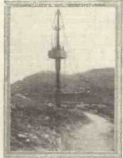
Showing the manner in which the tall steel masts are built up section upon section.
