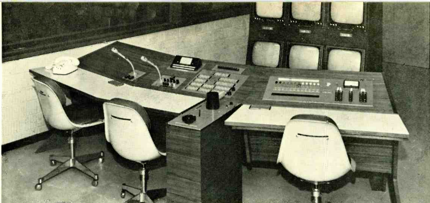
Fig. 8. Studio C control room.
