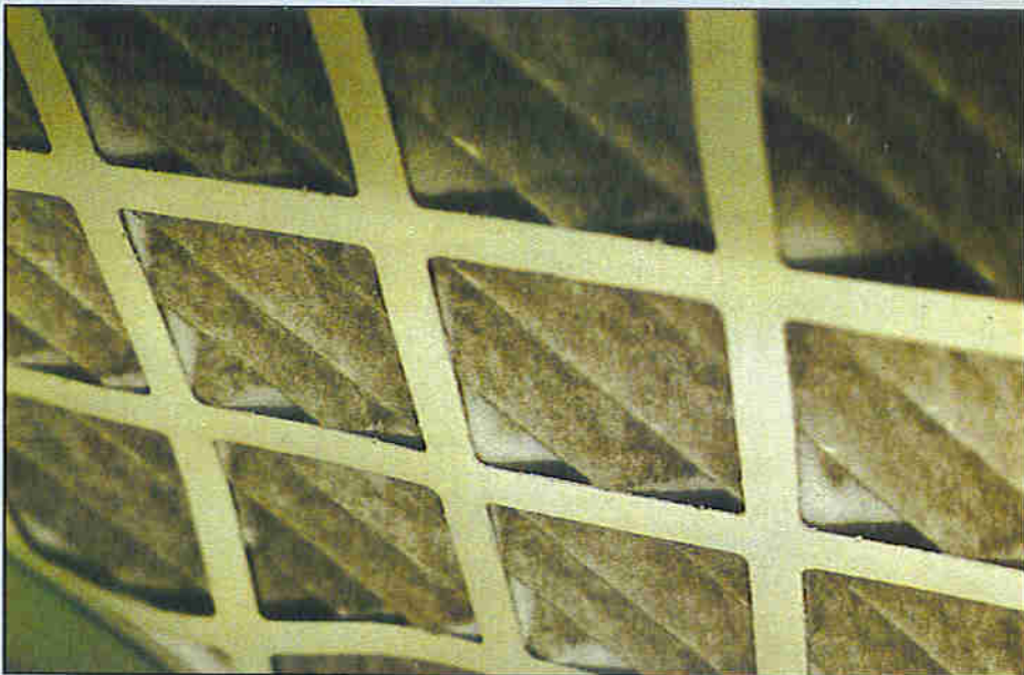
Blocked air filters reduce the efficiency of cooling equipment.
