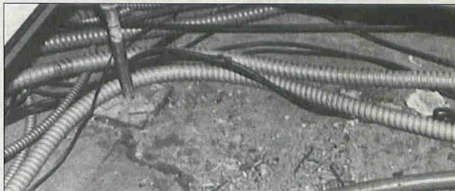
Dust and debris can be easily blown into equipment by differences in air pressure caused by air-conditioning and ventilation equipment.
