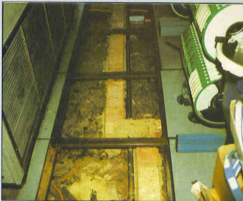
This subfloor is just waiting to cause problems!
