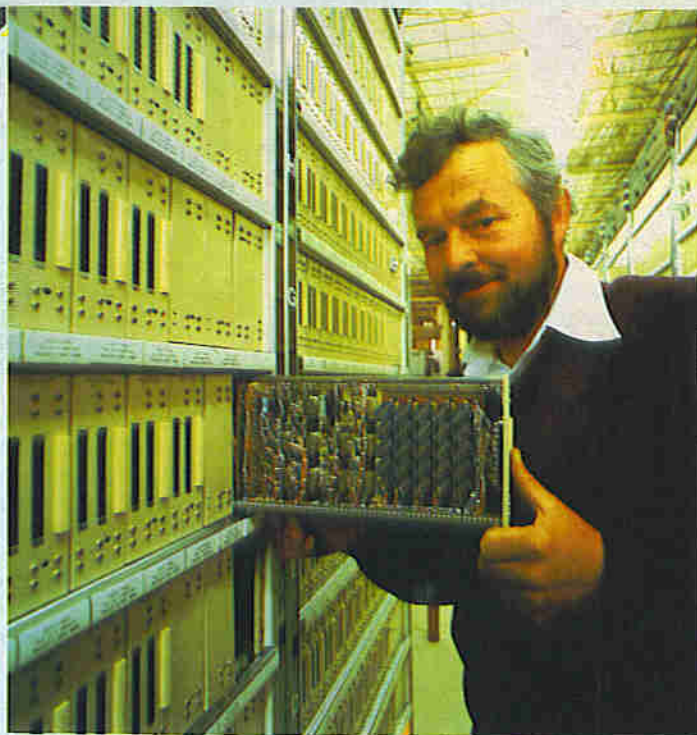
Photo 2. Front of System X rack with a card being removed.
