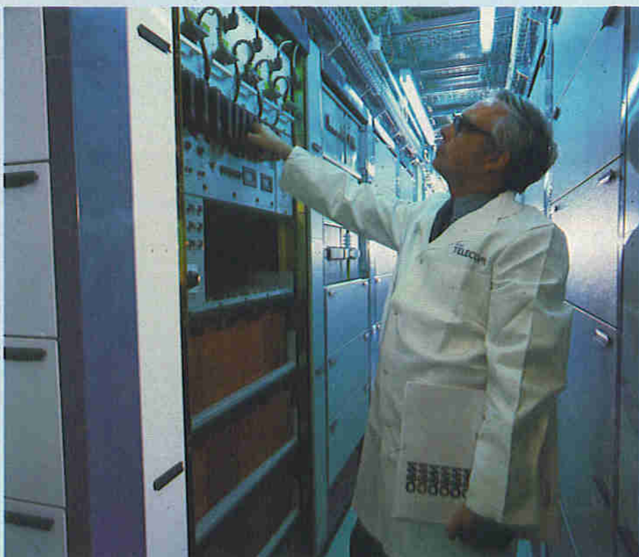
Photo 1. Front of System X rack cabinets.
