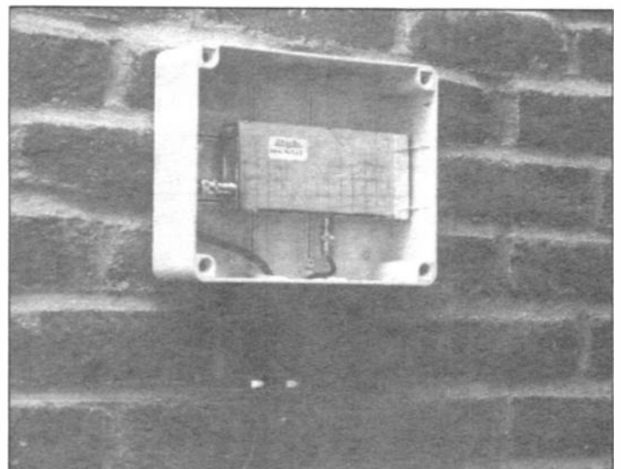
Down Converter mounted on a wall.
