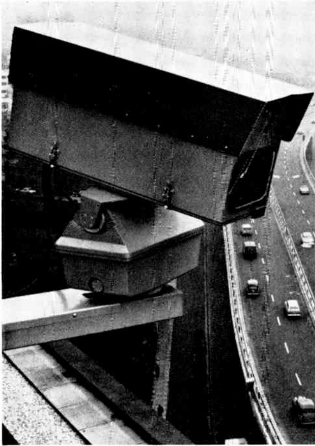
Fig. 1. Shown here is one of the three remote closed-circuit television cameras which overlook the elevated motorway
