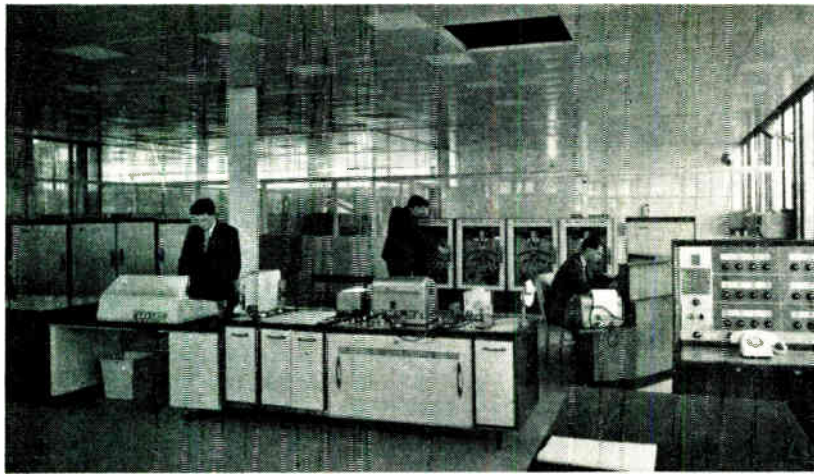
General view of one of the computing systems in the computer room at the Spencer Works of Richard Thomas & Baldwins Ltd. The computer is housed in the cabinets on the left, the film store is at the back and the programmer's console at the front. The control console is on the right and is shown in greater detail in another photograph
