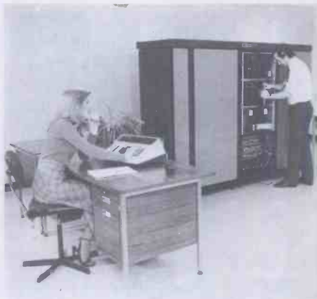
Plessey PDX 800 line electronic digital exchange (PABX) — an electromechanical equivalent would have totally filled the room.
