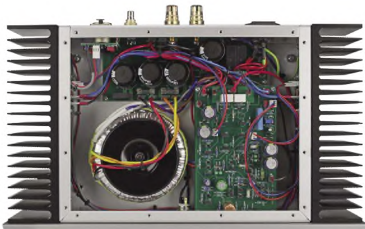
A large toroidal mains transformer (bottom left) feeds smoothing capacitors on the supply board (above).
