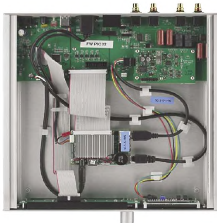
To the left of the analogue, gold plated input and output sockets (at right) sits a large LAN (Local Area Network) socket with connection into the processor that facilitates computer setup.
