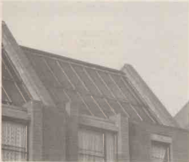
Solar panels (used for domestic water heating) incorporated into the roof of a house in South East London. (Martin Bond/Science Photo Library)
