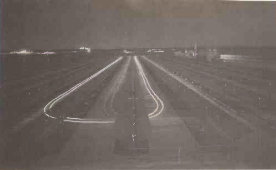
Mirrors of the Luz Solar Power Station seen in moonlight. The 1.5 million mirrors concentrate the sun's light onto narrow tubes containing synthetic oil. The oil is then fed to a heat exchanger where it boils water to provide steam for turbines, this installation can generate 150MW of power. (Roger Reismeyer, Starlight/Science Photo Library)
