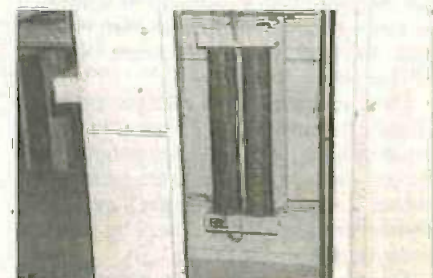
The "neutral resistor" is designed to limit fault currents in the generator. It connects between the star point and earth.
