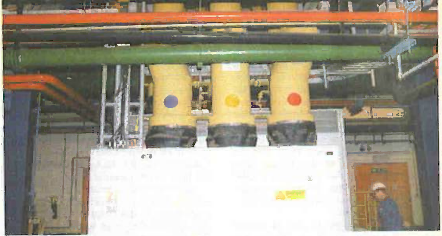
A circuit breaker unit connected to the gas turbine. Notice the colour coding "spots".
