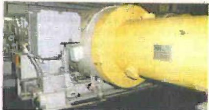
A gas-filled circuit breaker, rated at 17.5kV 10,000A, connected to the gas turbine generator.
