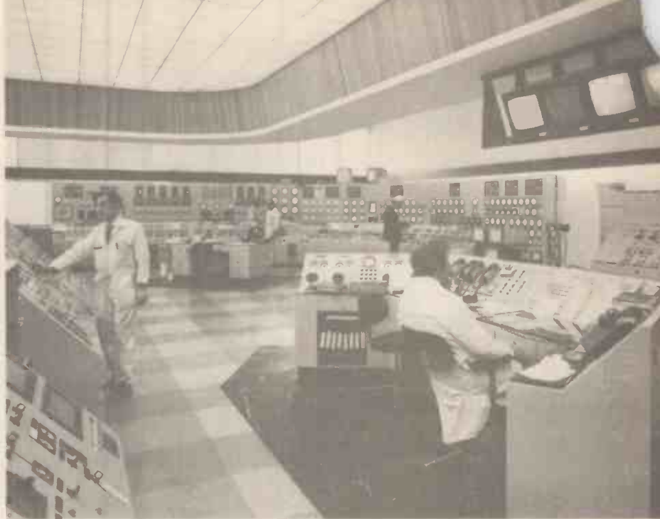
The main control room at the coal-fired Ratcliffe-on-Soar power station.
