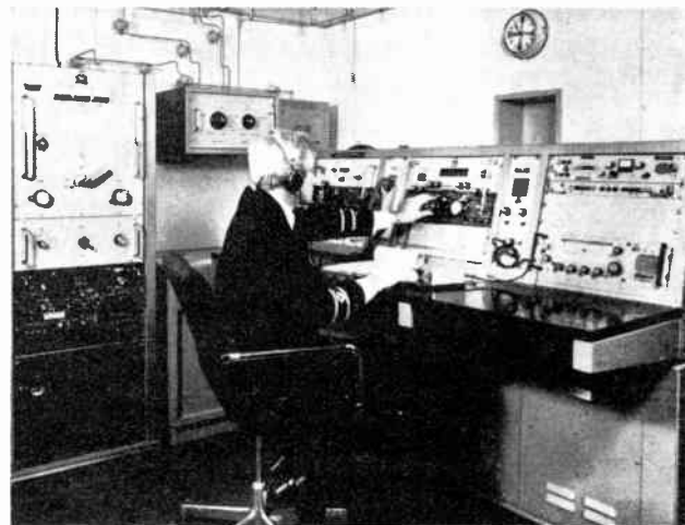
Fig. 1. General view of radio room showing main communications transmitter with open type aerial feeder and a communications console.
