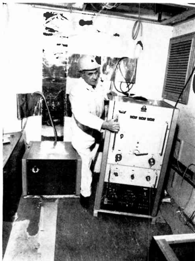
Fig. 2. Interior of radio room showing 30 cm wide copper earthing strips fixed to the bulkhead prior to installing the transmitter.
