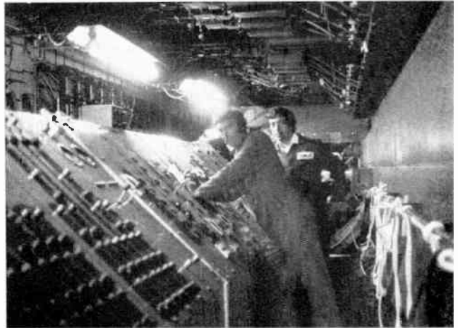
8. Remote control consoles on the control ship
