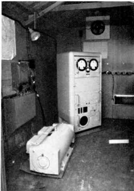
Fig. 4. The control console and motor alternator.
