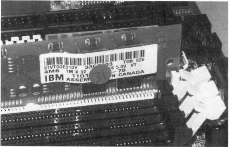
Fig.6.9 In this close-up view it is apparent that the SIMM is not properly in the socket at one end
