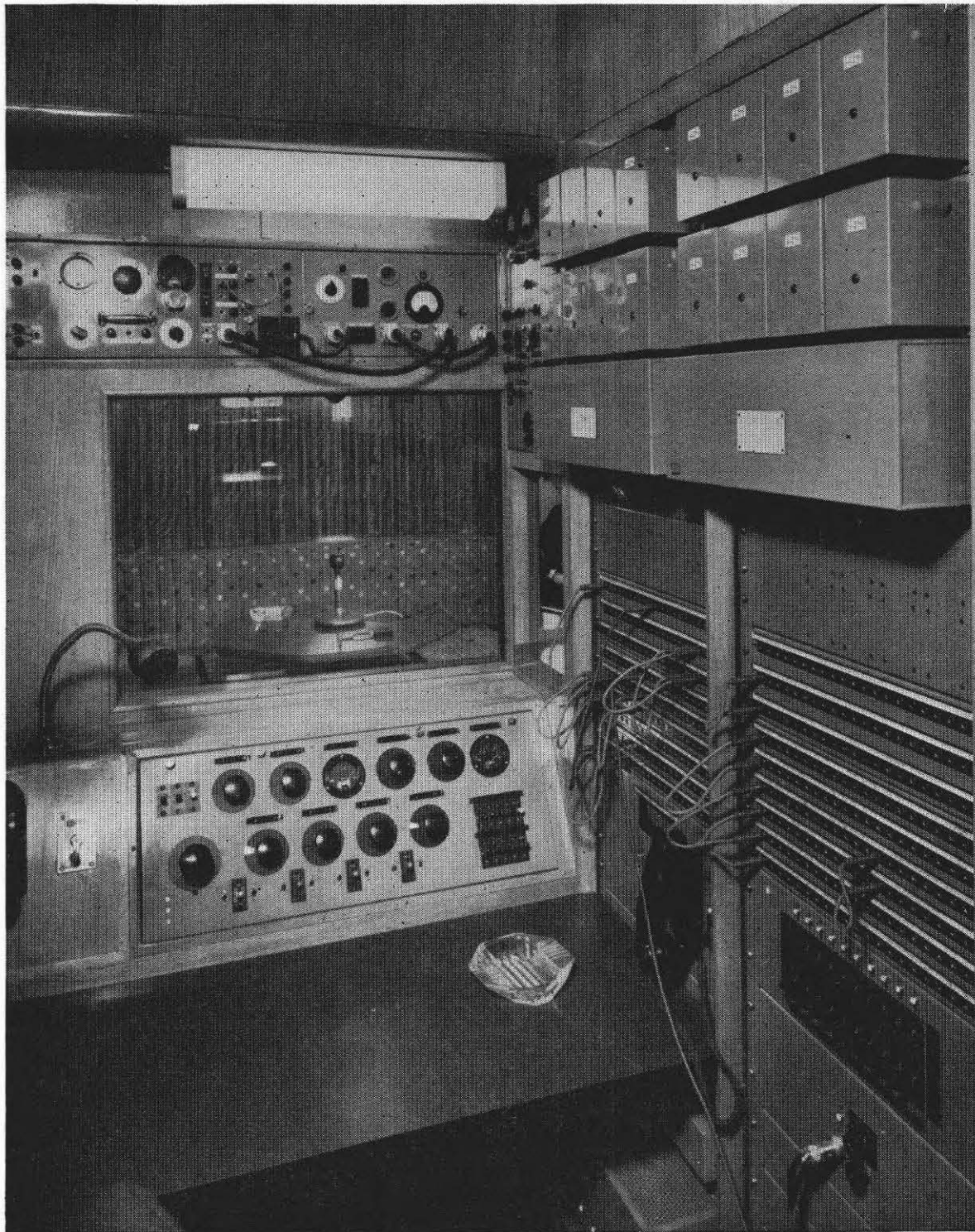
Fig. 7 — The engineering control position showing desk, rack-mounted equipment, and the studio beyond. Note reflection of man in entrance lobby in mirror to right of studio observation window
