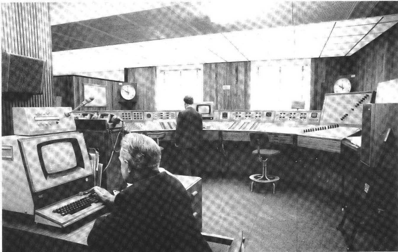
Fig. 1 The control desk position is designed for standing operation during periods of high activity. In the foreground can be seen the supervisory terminal
