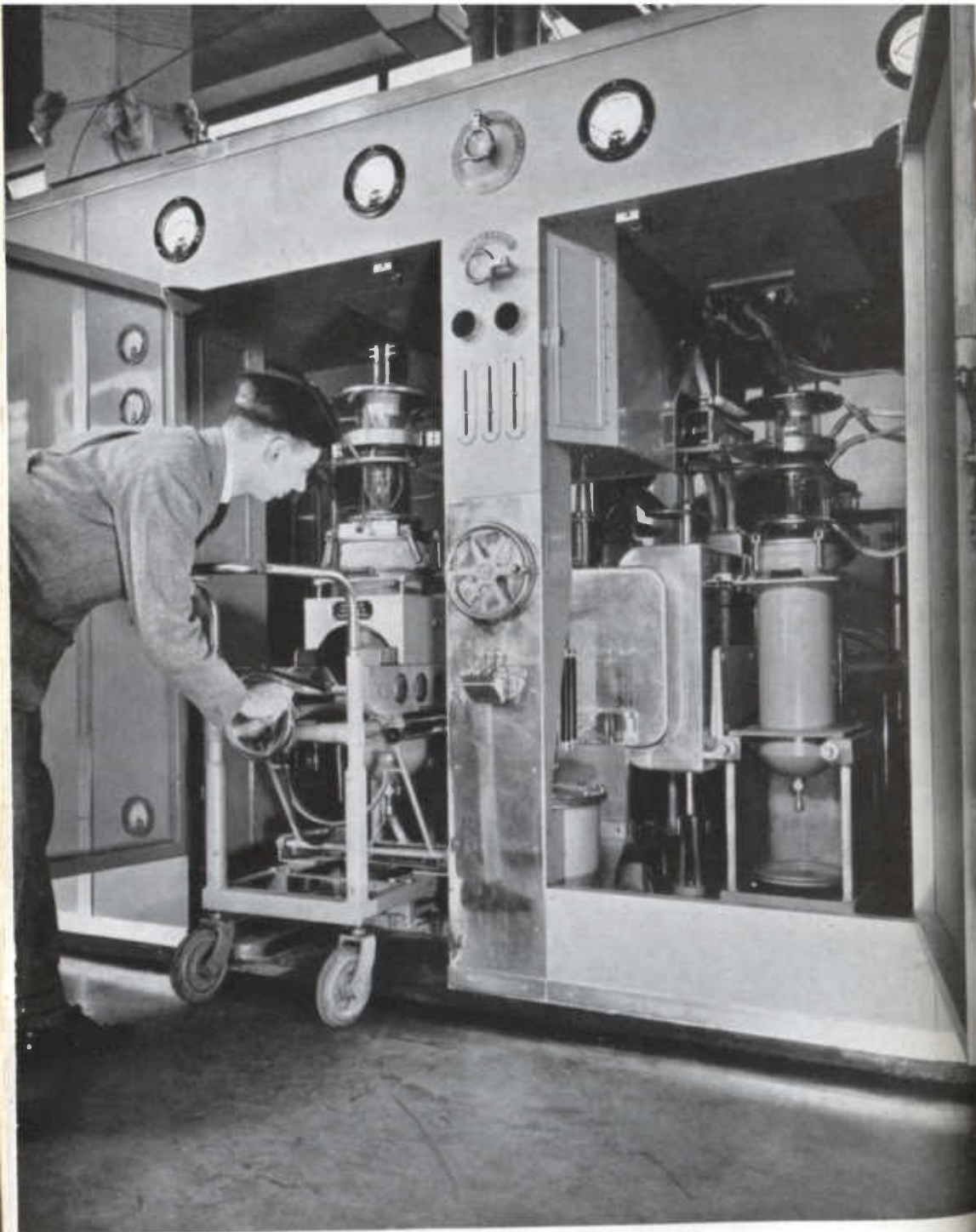
Large water-cooled valve being wheeled into position
