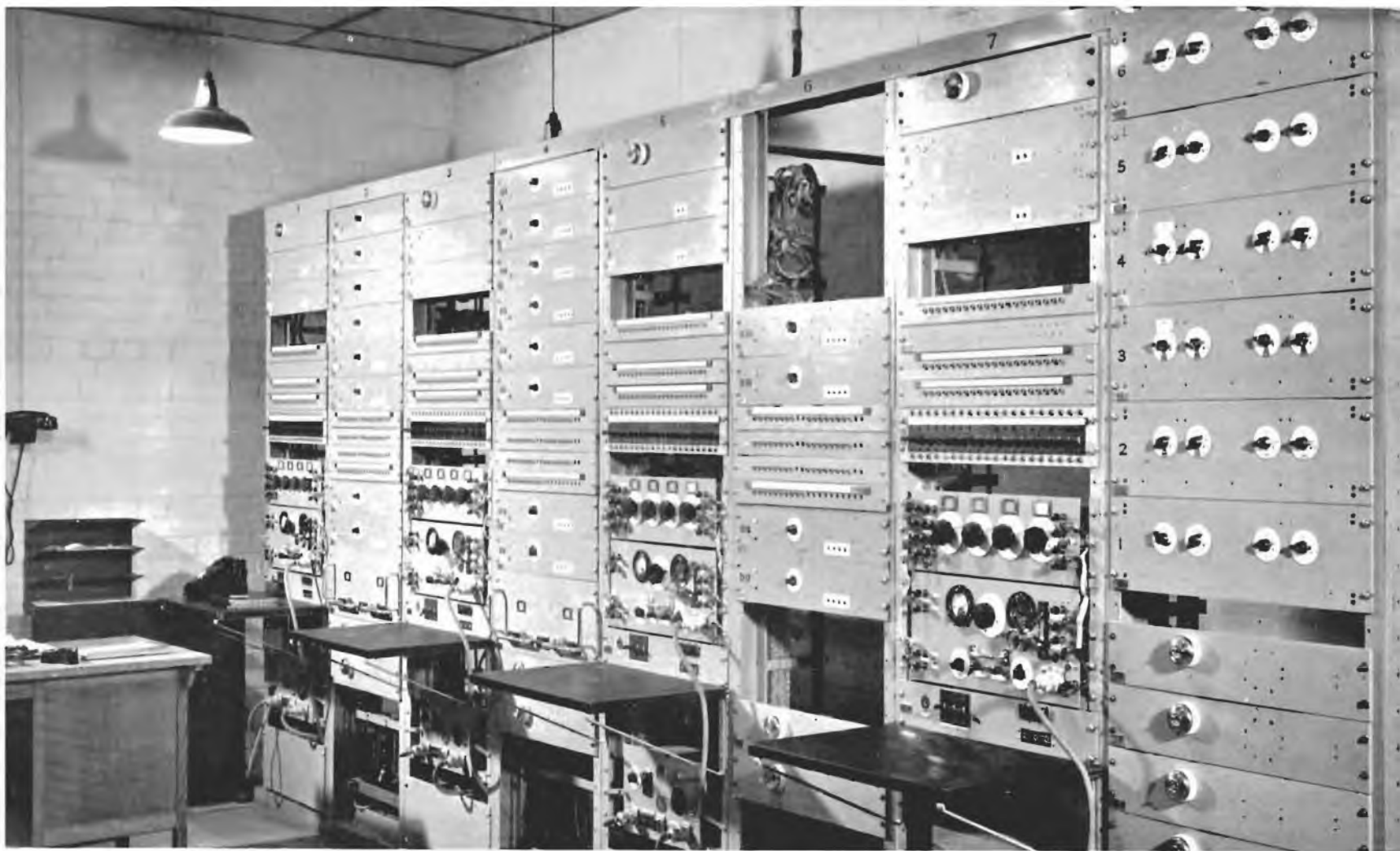
Control position bays in a wartime control room Plate XV
