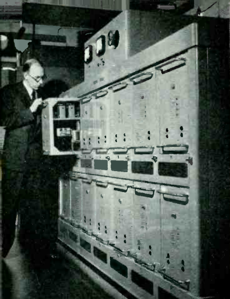
MULTI-UNIT TRANSMITTER, BRIGHTON, designed for unattended operation and remote control.
