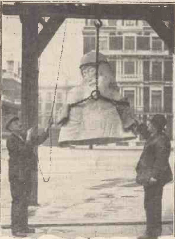
A huge 10-ft. sculpture portraying Prospero sending Ariel out into the world to discourse unearthly music is being erected above the entrance to Broadcasting House. The work is by Mr. Eric Gill, and is executed in Portland stone
