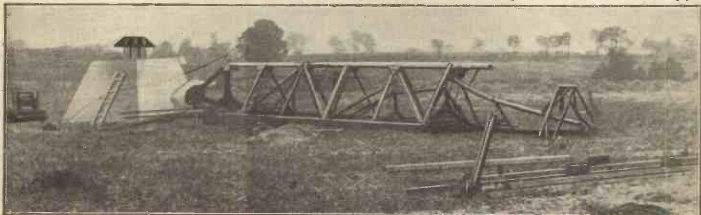
The mishap at West Regional. One of the new steel masts crashed recently when partly erected, with fatal results. The supports broke and it collapsed from the huge insulating base, killing one and injuring two.
