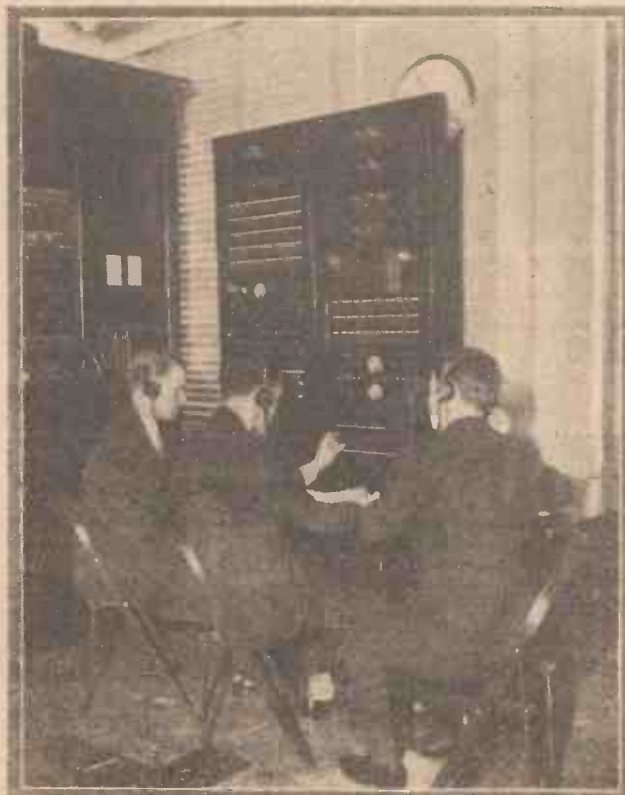
American control-room practice differs from ours and here engineers are seen at one of the switchboards in the National Broadcasting Company's main control room in Fifth Avenue
