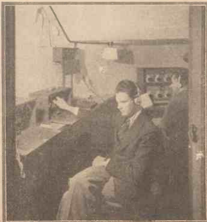
B.B.C. engineers at the balance and control point during a broadcast. The dual sets of panels control the volume, the number of microphones in circuit and the microphone amplifiers
