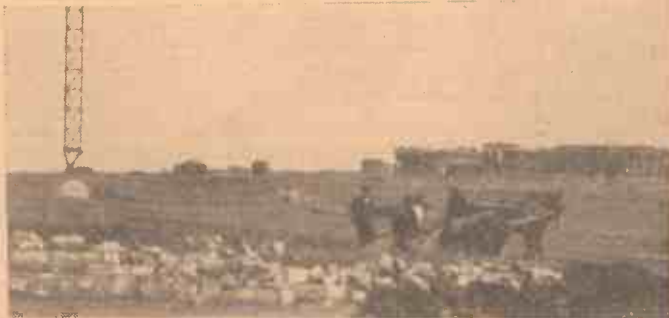
Great progress has been made with the Slaithwaite station, and this picture taken recently shows one of the masts in the course of erection. The building is nearly ready for the installation of the bigger plant such as the H.T. generators
