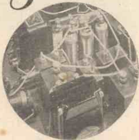
Close-up of filter and coupling arrangements of the amplifier
