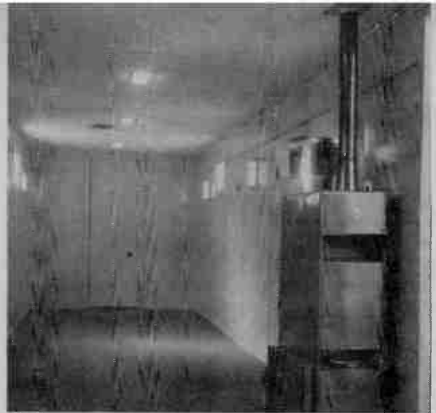
Figure 3. Interior view ready for equipment installation.
