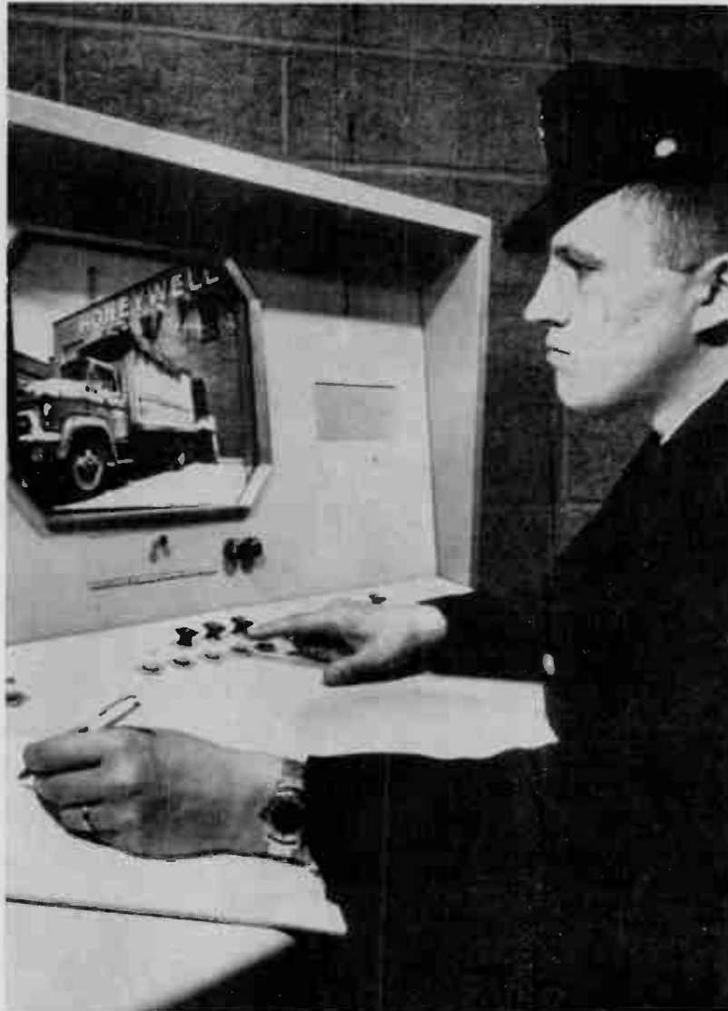
Nerve center of a new building protection and security system designed by Minneapolis-Honeywell Regulator Company is this centralized console. With it, a single guard can supervise an entire building security system.
