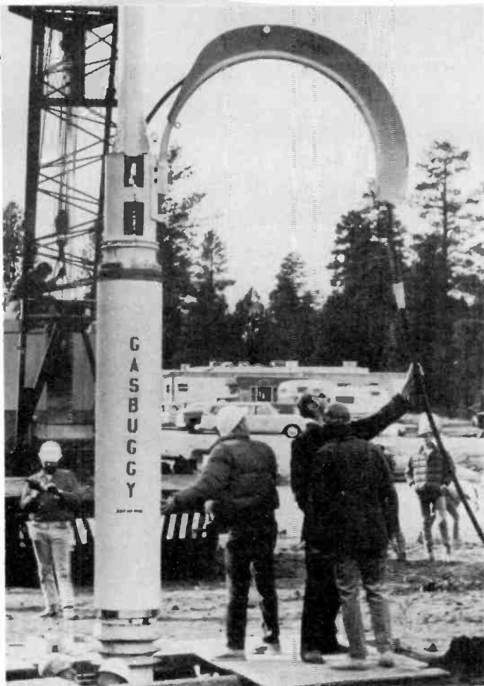
A canister containing the 26-kiloton explosive for Project Gasbuggy is lowered to a depth of 4240 feet and covered to within 50 feet of the surface with cement. Gasbuggy was an effort to determine the feasibility of recovering natural gas using nuclear explosive techniques. Photo courtesy of U.S. Department of Energy.
