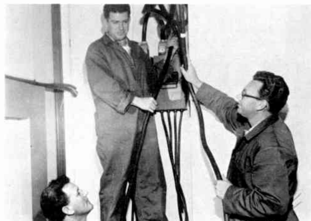
Lights for the Media Theatre being installed by Archie Kay, George Smith and Julien Madaire.
