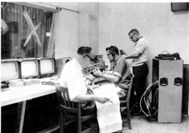
Installing video switcher in TV Studio 1: Eugene Wacholz, Stan Dellagana and Walter Kulish.
