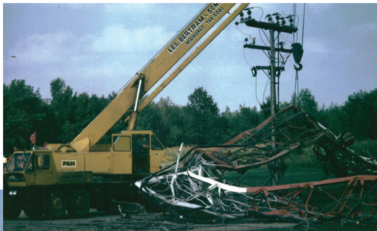
Clearing the crumpled 1,000-foot tower after the crash
