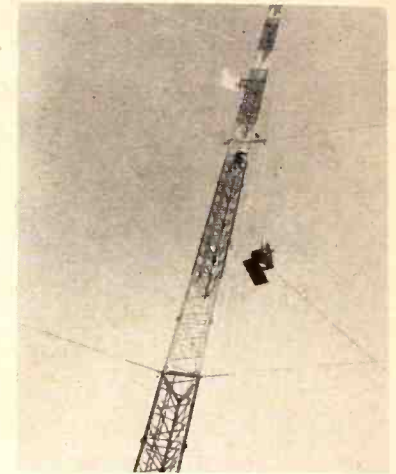
THE MICROWAVE UNIT which enabled CKOS-TV, Yorkton to broadcast the World Series to its viewers is seen here being hoisted into place on the station's 500 foot tower. Not yet on the microwave hook-up, CKOS installed the temporary unit as a special Canadian TV Week Promotion.
