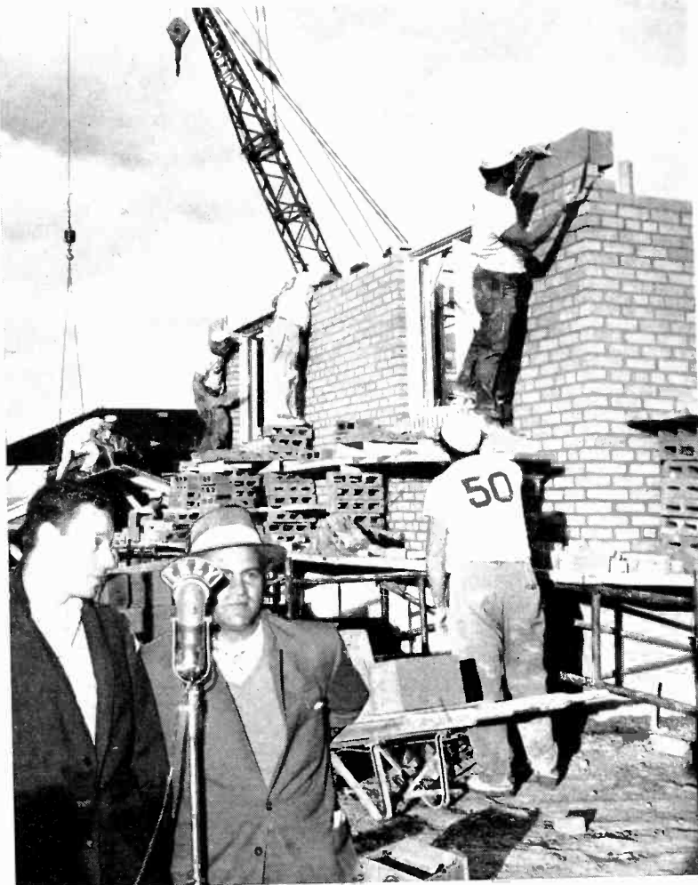
RICHARD SCOTT, STAFF ANNOUNCER FROM CKEY interviews Lawry Shankman (right), director of construction for Consolidated Building, while in the background work is rapidly progressing on the house.
