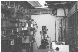
Photo 2: Central Equipment Room signal crossjumping, CFNY Radio
